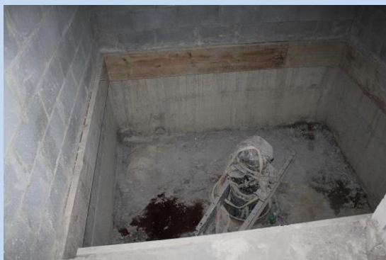
Temporary Electrician Helper Steps Into Unguarded Elevator Shaft And Dies - Kentucky (2016, April)
